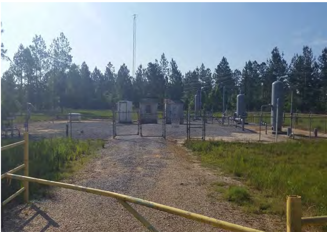
Photo 44: Gas facility on eastern side of LA-1088, north of I-12 interchange. Photo is looking towards the east.
