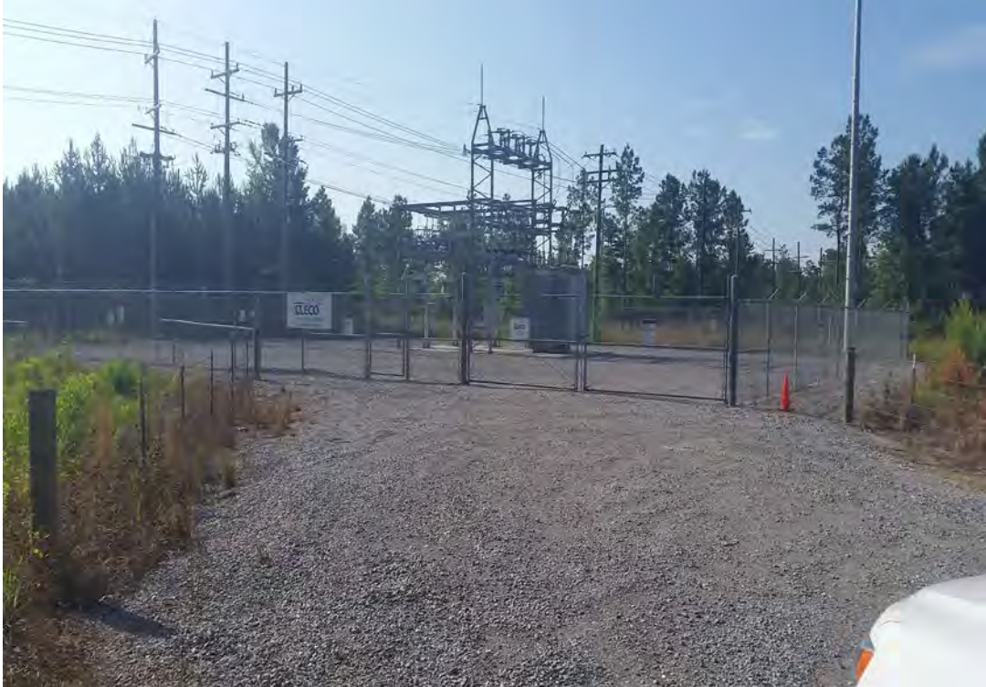
Photo 45: Electrical facility on eastern side of LA-1088 north of I-12 interchange.
